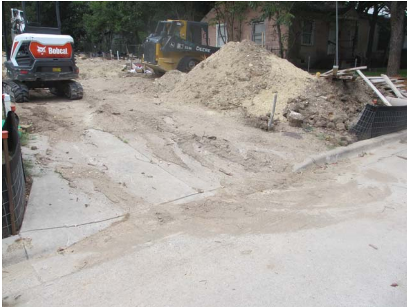
1404 Oxford - no erosion controls across entrance; considerable sediment in the street
