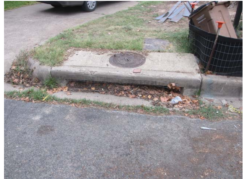
1300 Folts - sediment control screen on storm drain inlet is clogged and needs cleaned
