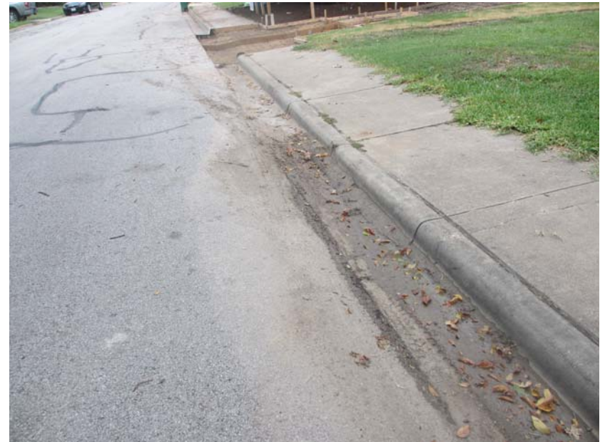
1811 Ashby - sediment deposited in gutter just downstream of construction site
