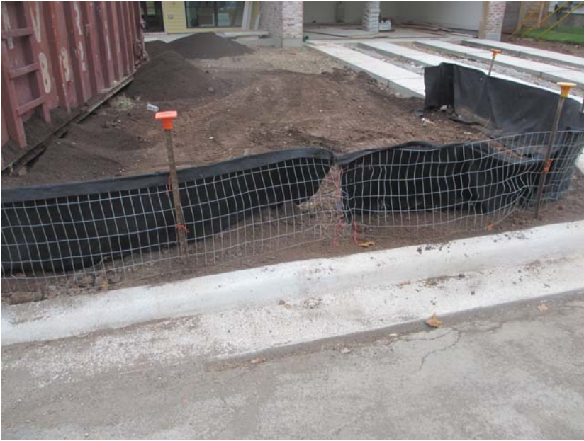
1300 Folts - silt fence not maintained; gap readily visible
