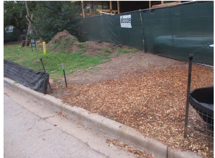
1206 Garner - gap in silt fence; while mulch may prevent soil under it from eroding, it is not contain runoff from upgradient
