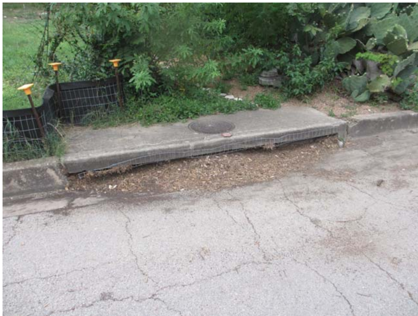
1813 Treadwell - sediment control screen on storm drain inlet is clogged and needs cleaned
