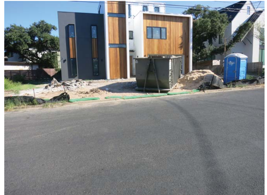
1401 Rabb (BSZ) - Mulch sock flattened and with gaps. No controls over or around dirt piles to prevent erosion.
