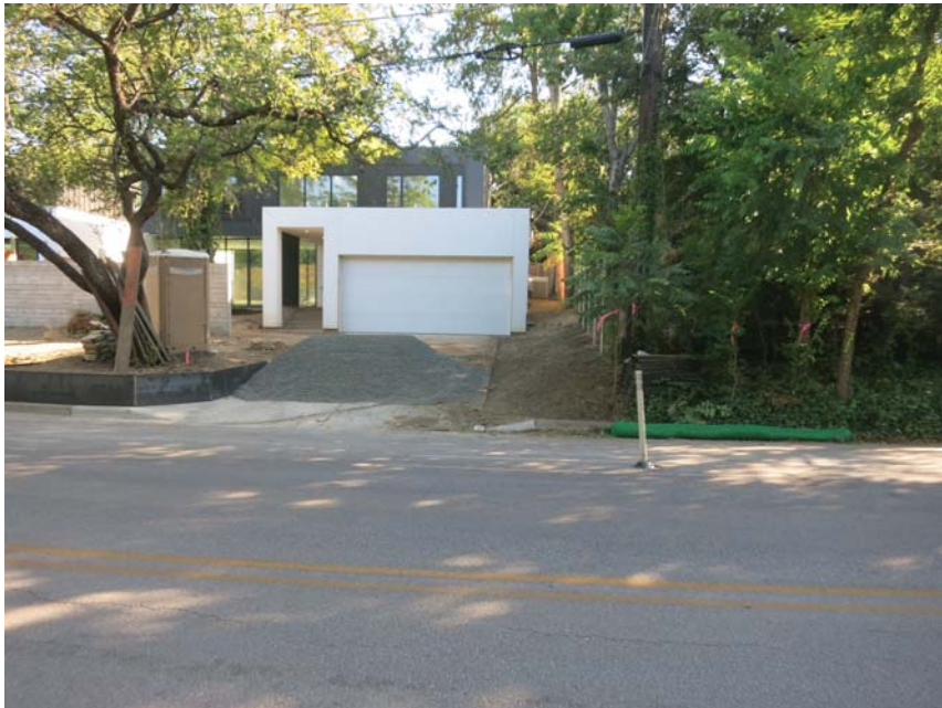
2005 Melridge (BSZ) - No controls to stop stream of water that will flow on steep slope down side of house, eroding sediment as it goes.
