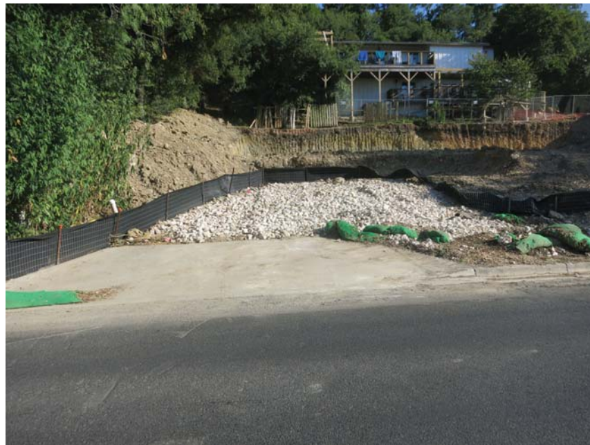
809 Azie Morton - Crushed silt fence with gaps under it. This site has high slope and unbraced excavation. It has the potential to be an environmental disaster if it rains. Flows to Barton Creek below BSP.
