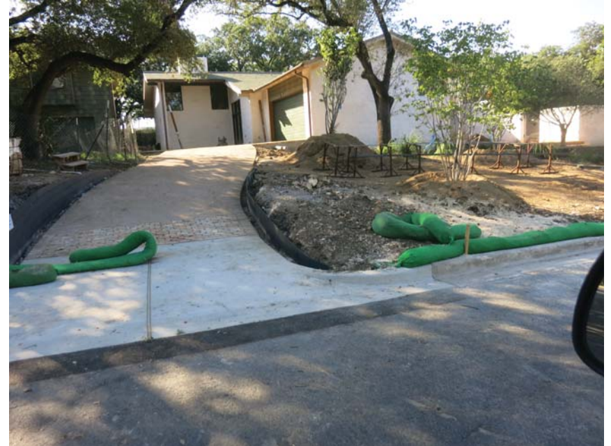
1912 Paramount (BSZ) - Steep slope without controls extending all the way across frontage will allow sediment to leave site.
