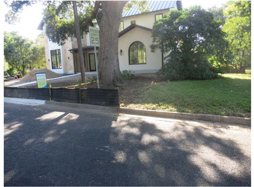
1804 Treadwell - Along Garner. The runoff with sediment will just flow along the silt fence and exit at the downstream end. All they would have needed to do is put in a j-hook to prevent the flow from exiting at the end. Without it, the silt fence might as well not be there.
