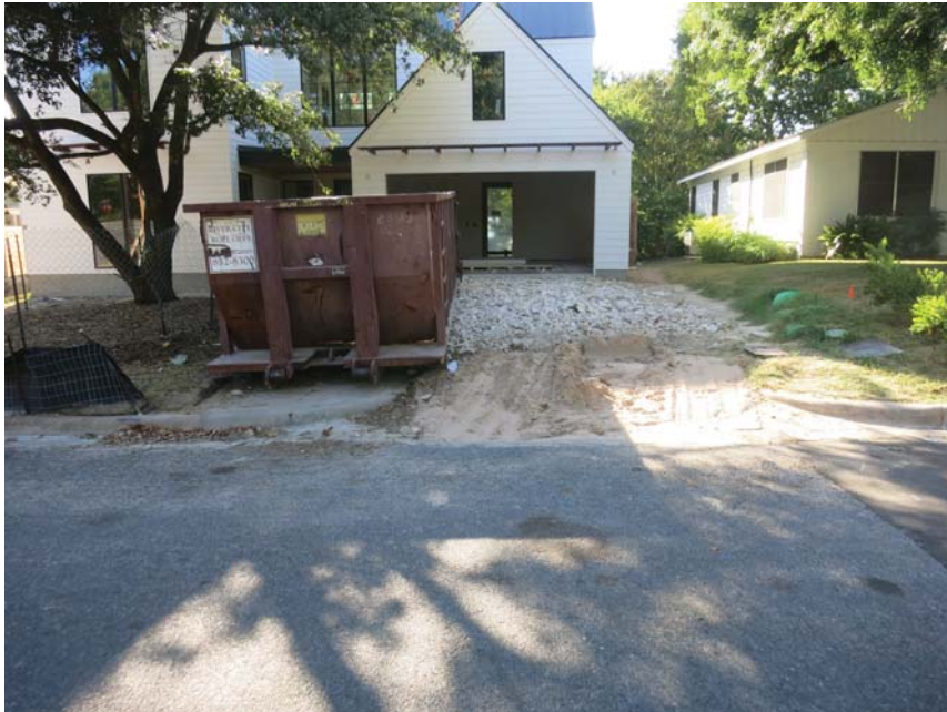
1208 Folts (BSZ) - Sand/dirt is piled at the end of the driveway and partially in the gutter where it will easily escape the site.
