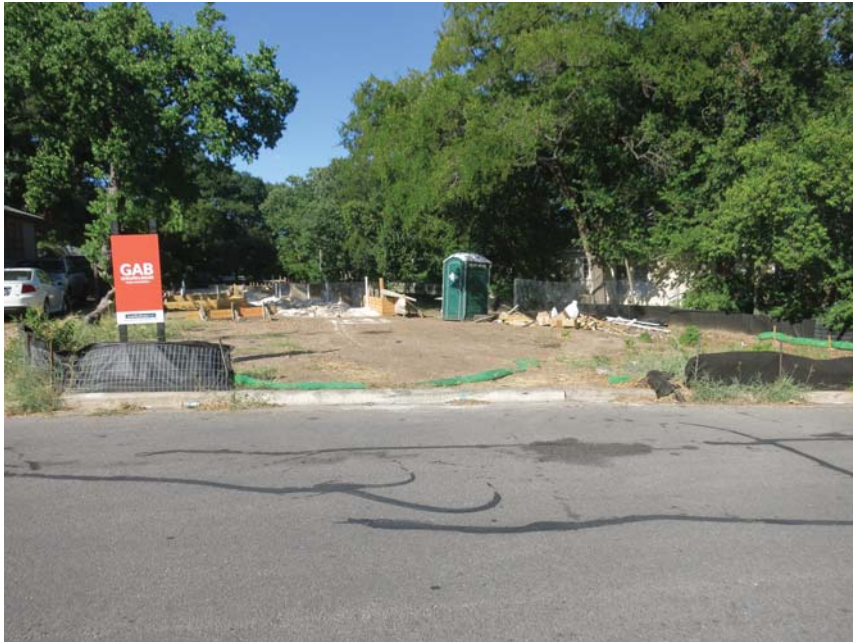
2104 La Casa - Flattened mulch socks (barely visible) will not prevent sediment from leaving the site.
