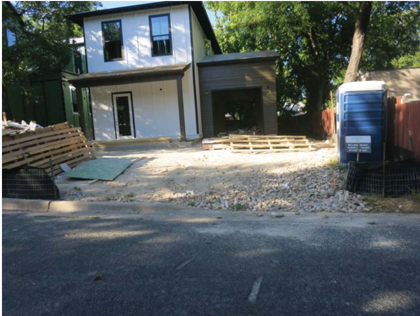
1718 Valeria - No controls across entrance. The silt fence on the left has no j-hook and will simply direct runoff to the street.
