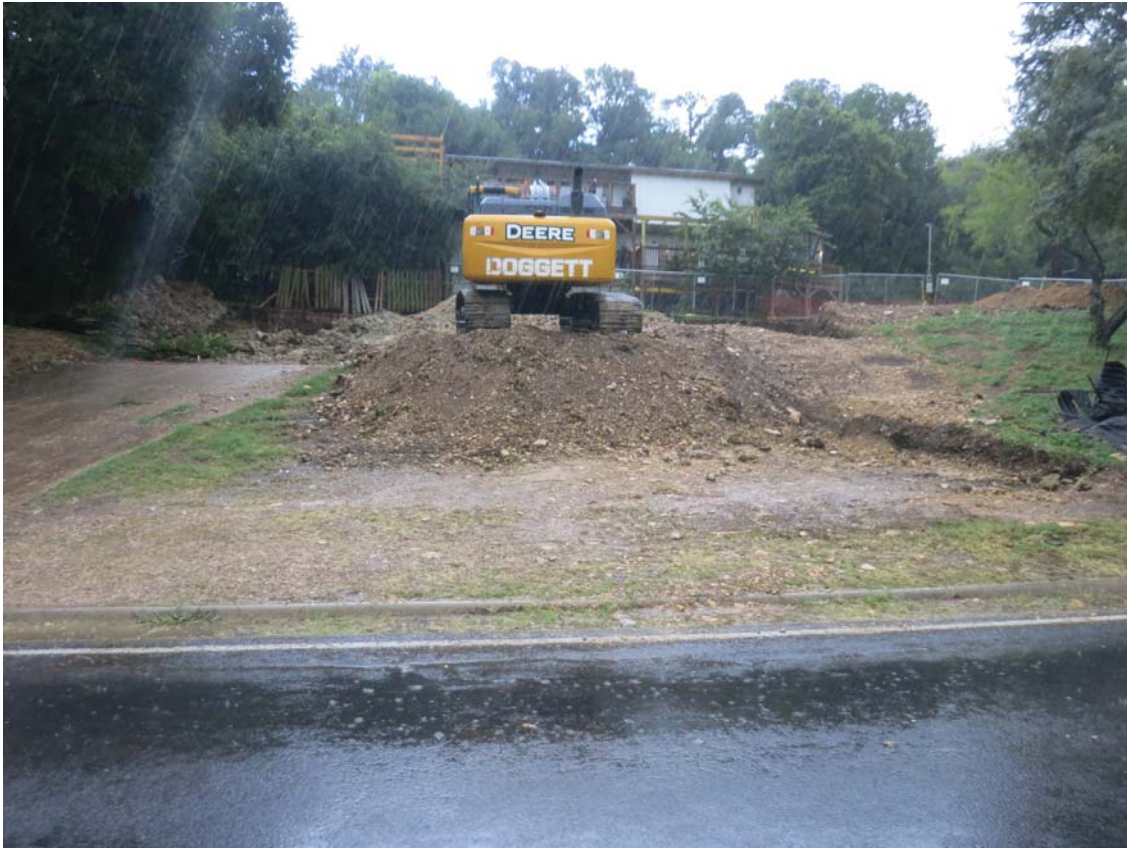
809 Azie Morton - No erosion controls.
