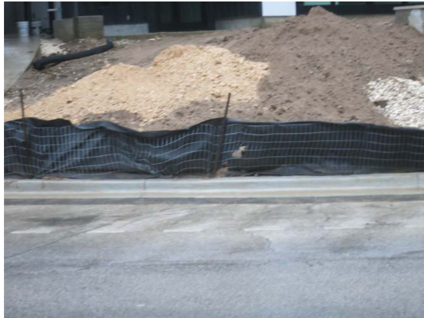
Holes in silt fence.
