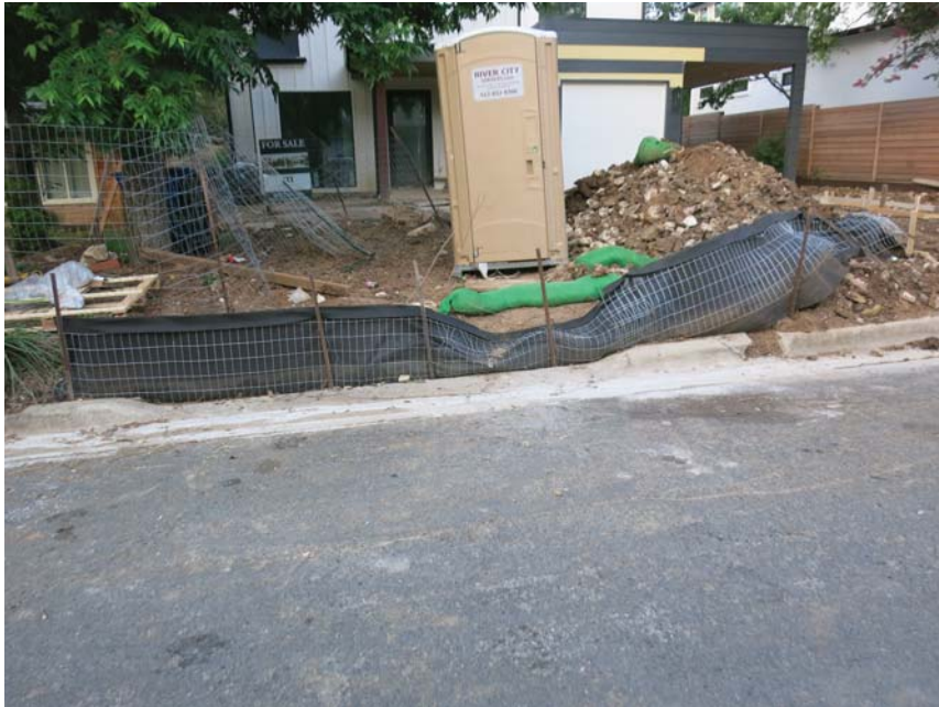
2109 Peach Tree - Crushed silt fence. No j-hook on left end.
