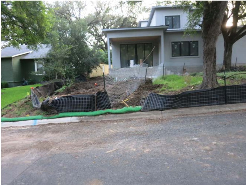
Crushed silt fence at corner. Gap in silt fence without j-hooks. Mulch socks do not have j-hooks.
