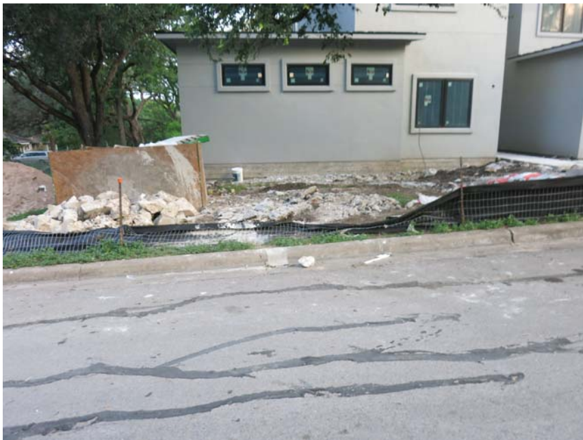
Crushed silt fence.
