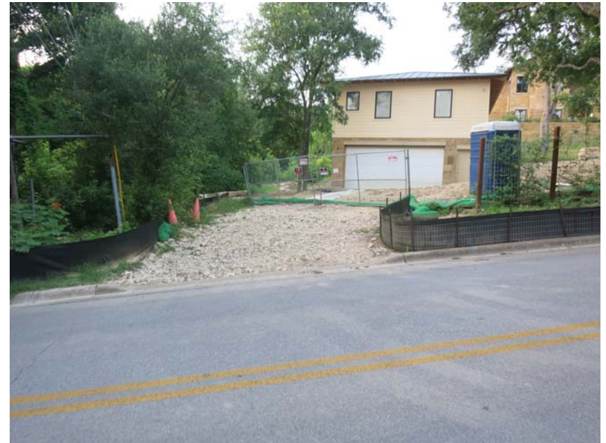
1113 Azie Morton - Water funnels down driveway with only one mulch sock row. Slope requires more. Muddy water floods off of this driveway whenever it rains.
