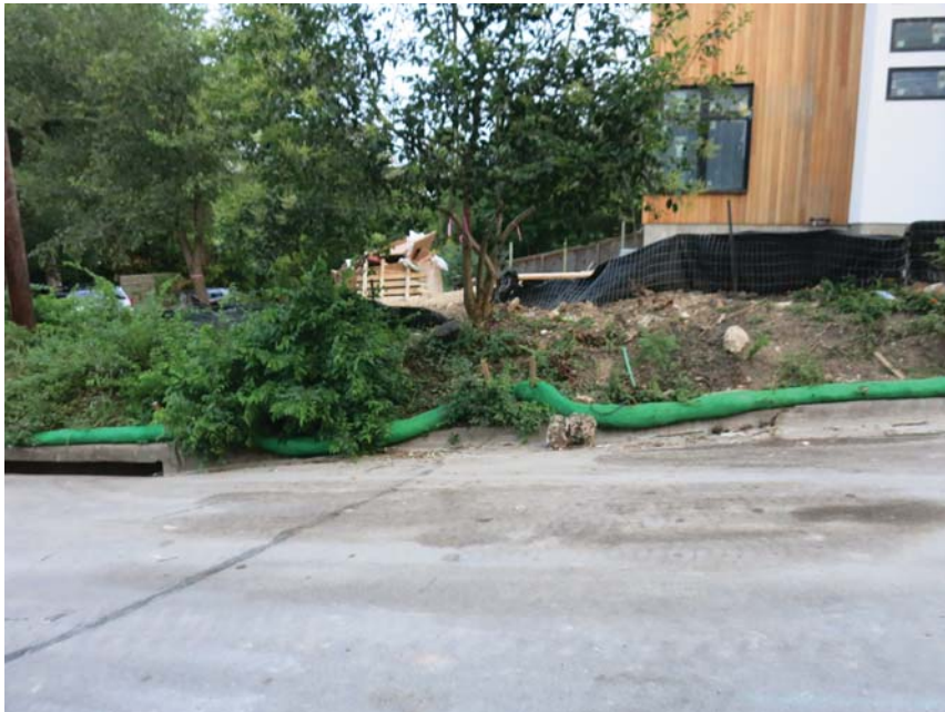
Mulch socks are not allowed on a slope this steep.
