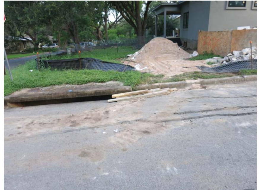
No controls for pile of sand which has crushed silt fence. Sediment visible in street. Storm drain inlet immediately adjacent.
