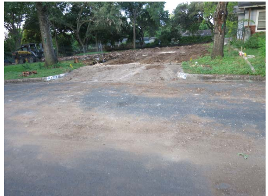
1717 Norris - No controls along front. Substantial amounts of sediment and dirt in street.
