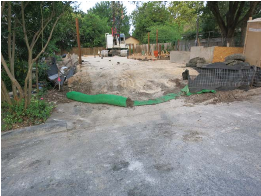
2103 Peach Tree - Mulch sock completely flattened and totally ineffective. Not staked. No j-hooks on mulch socks or silt fence.
