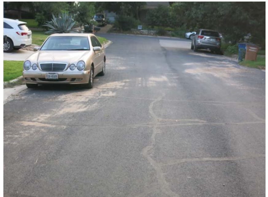
Sediment downstream of site that has never been swept up.
