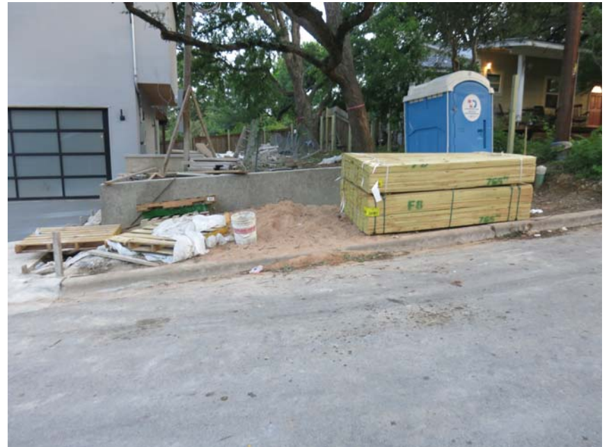
No controls for pile of sand which is immediately adjacent to gutter.
