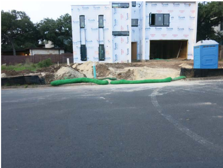
1401 Rabb - Gaps in mulch socks. Not staked. No j-hooks on mulch socks or silt fences.
