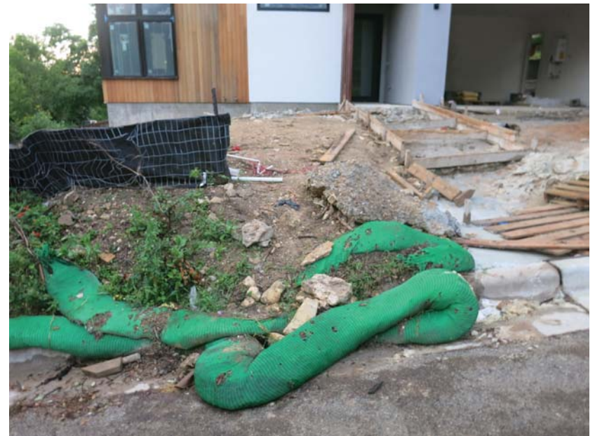
mulch sock with soil overtopping them will not stop erosion
