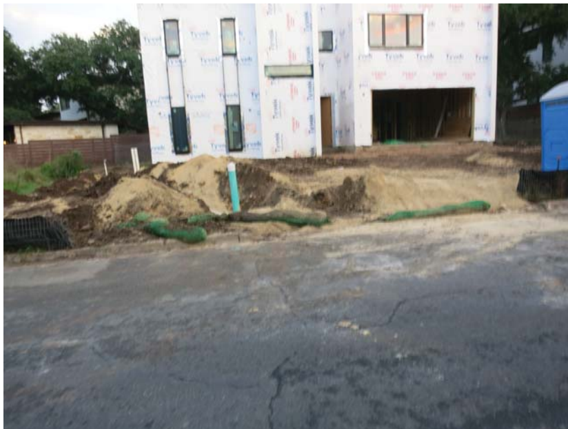
1401 Rabb - loose aggregate with haphazardly placed mulch socks with gaps that will not prevent erosion
