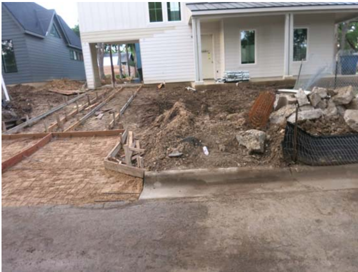
along De Verne - no controls for sand in driveway and no controls between driveway and silt fence
