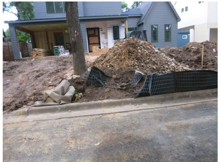
along De Verne - dirt piled on top of and over silt fence
