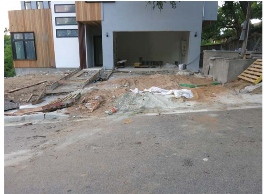
no controls; loose sand and powdered cement (gray) will erode directly into gutter when it rains
