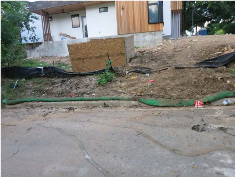
flattened silt fence and flattened mulch socks have no hope of preventing erosion
