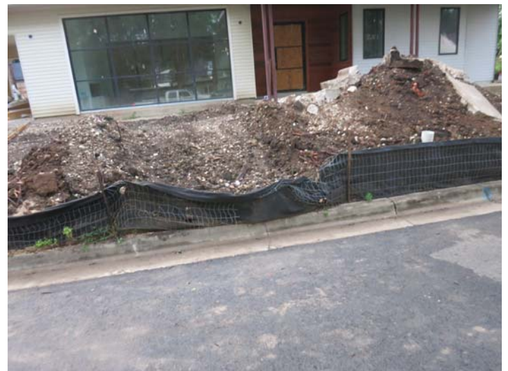
along Paramount - dirt piled up to top of partially crushed silt fence; silt fence has a hole in it
