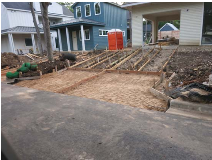
along Paramount - no controls for sand in driveway and crushed silt fence to the right of driveway
