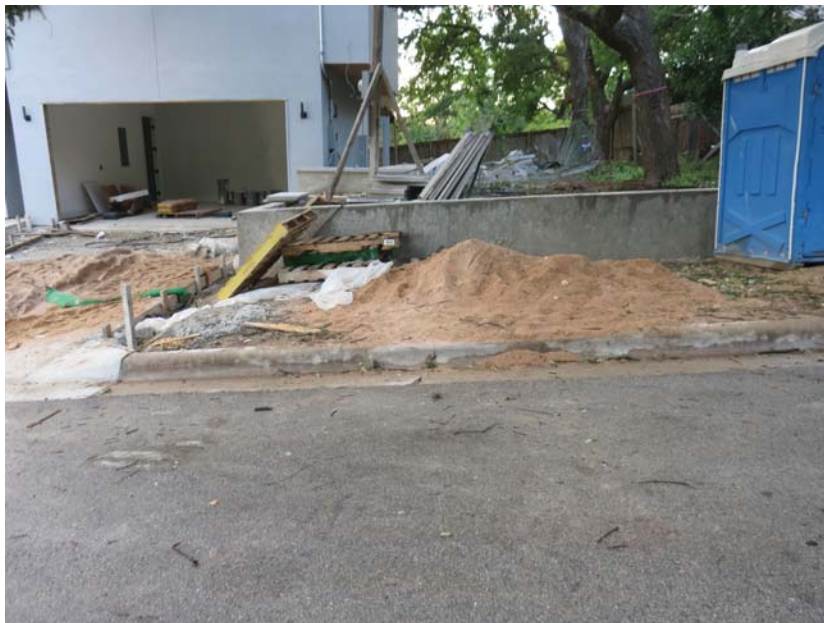
loose sand with no controls and sand in gutter
