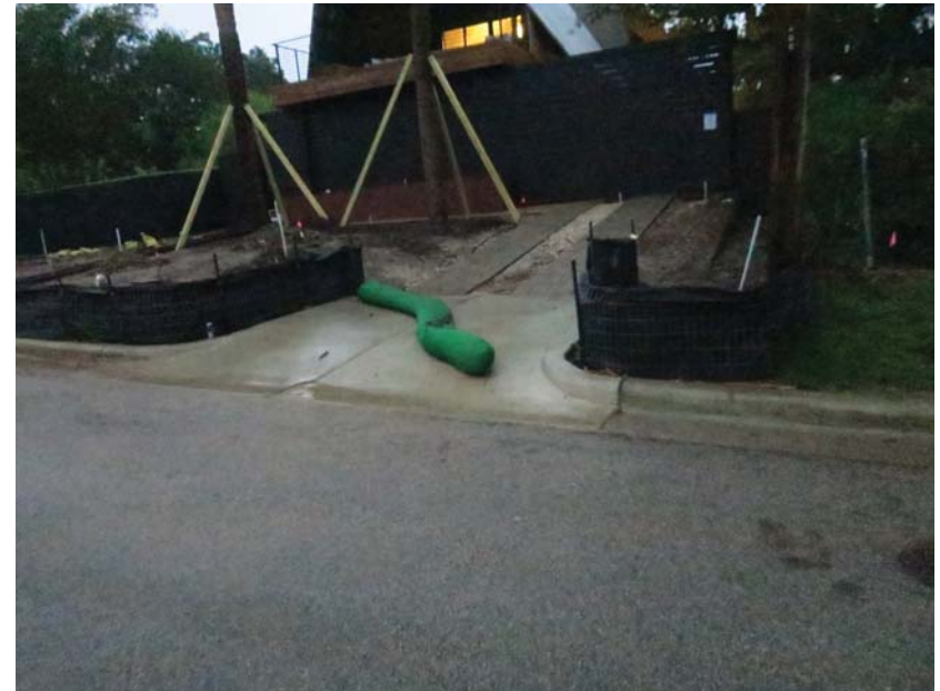
8640 Garner - mulch sock not secured; as a result, runoff and sediment is just directed down the driveway and into the gutter
