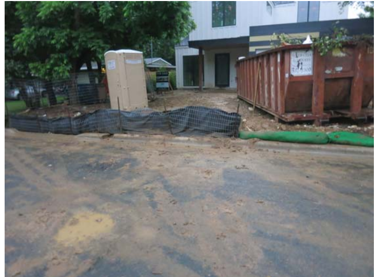
bottom of silt fence not towed-in; sediment escaping site
