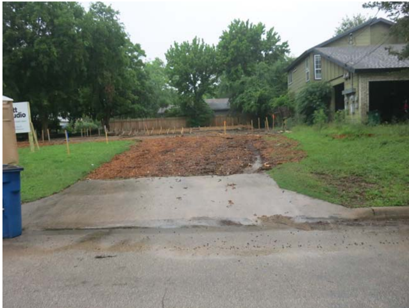
1712 Goodrich - placing mulch on bare ground with this much slope is ineffective; it simply washes off with the sediment; more controls are needed
