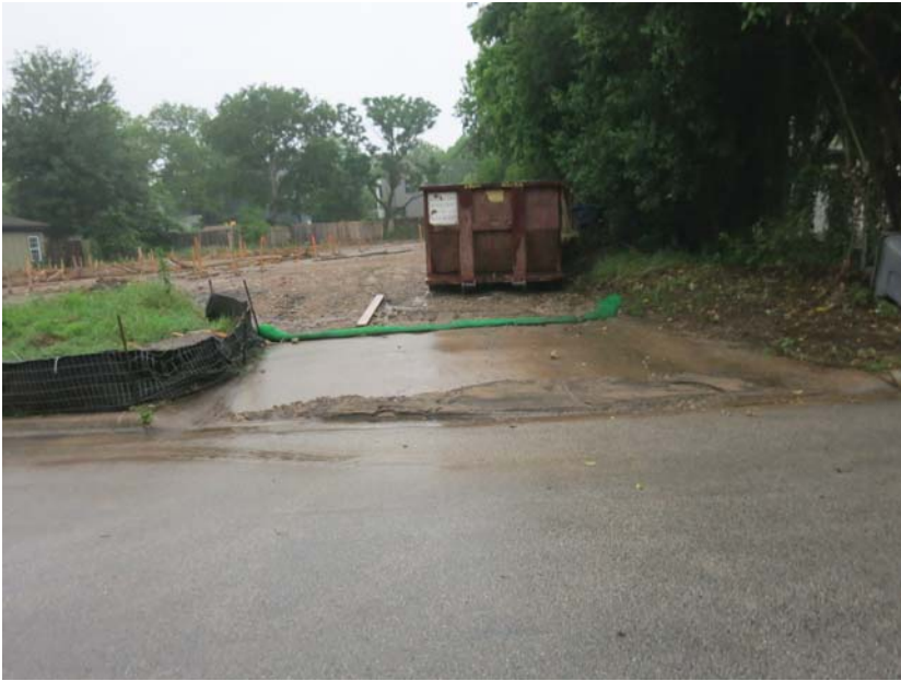
1706 Goodrich - flattened mulch sock; sediment leaving site, some much of which still remains in the gutter
