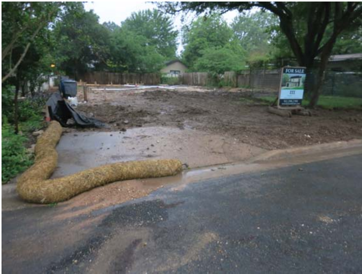
straw waddles are not acceptable controls and this one is mostly ineffective
