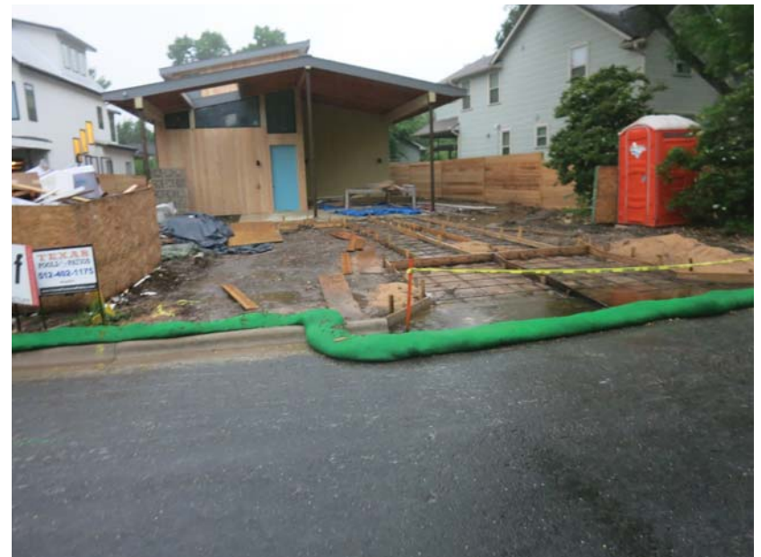
1811 Collier - flattened mulch socks on left side do not prevent sediment from leaving site; much socks in street not secured; heavy rain will wash them down the street
