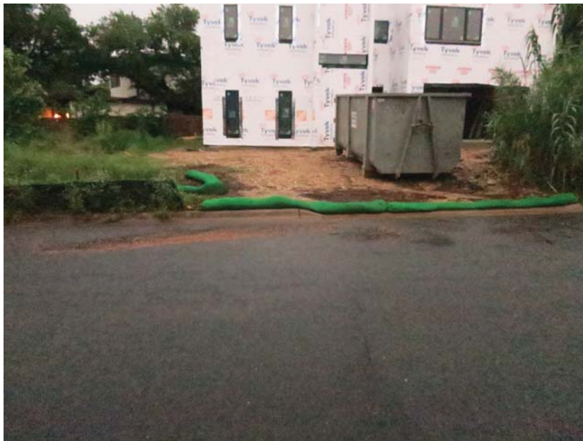
1401 Rabb - gaps between silt fence and mulch sock; mulch socks are not effective in prevent sediment from leaving site; the runoff overtops the controls as evidenced by sediment in street
