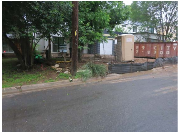
silt fence does not have j-hook on left end allowing runoff to escape after it flows along the silt fence
