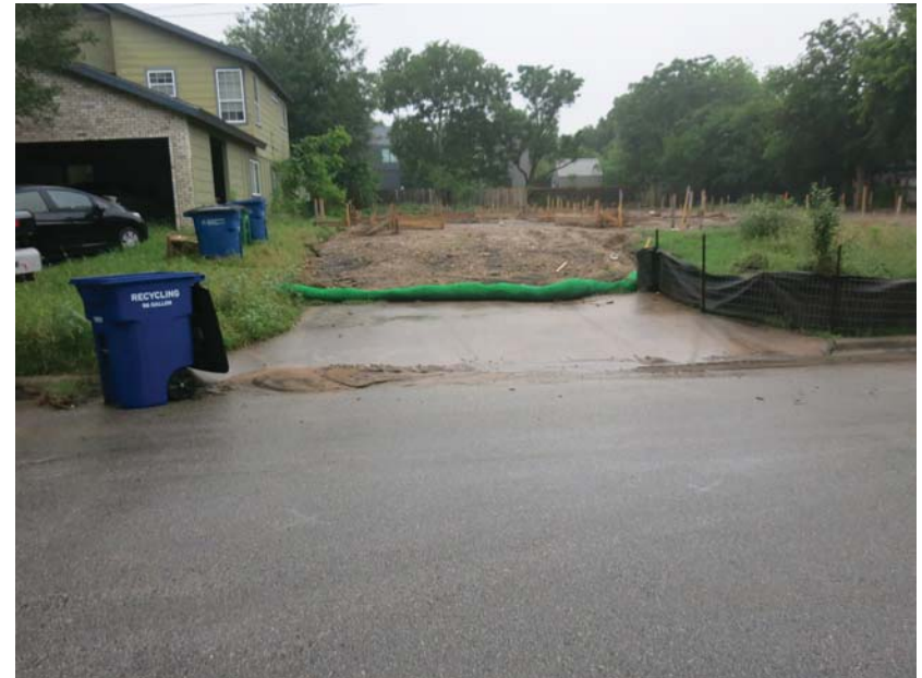
1708 Goodrich - mulch sock not preventing sediment from leaving the site; sediment visible in gutter
